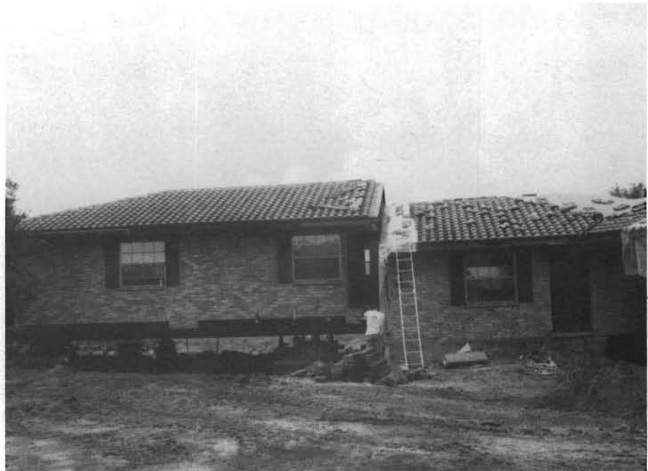
One section of the house has been raised preparatory to inserting the wheeled dollies.
