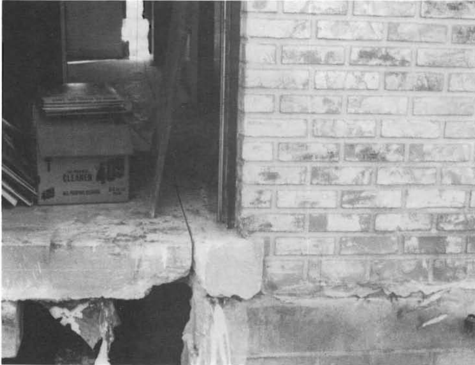
This large home had to be moved in several sections to accommodate the restrictions of the travel route. Here the slab has been cut with a street saw.
