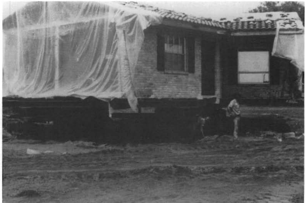
Plastic sheeting covers the open end of the room for weather protection during the move.
