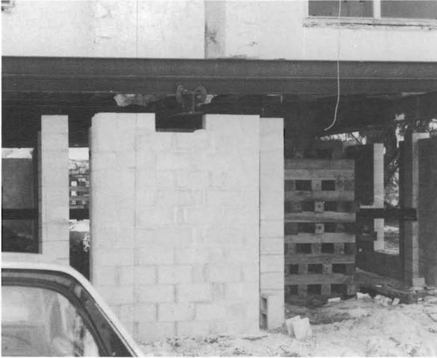
The foundation for the fireplace has been partially constructed. The temporary cribbing supporting the structure is visible in the background.
