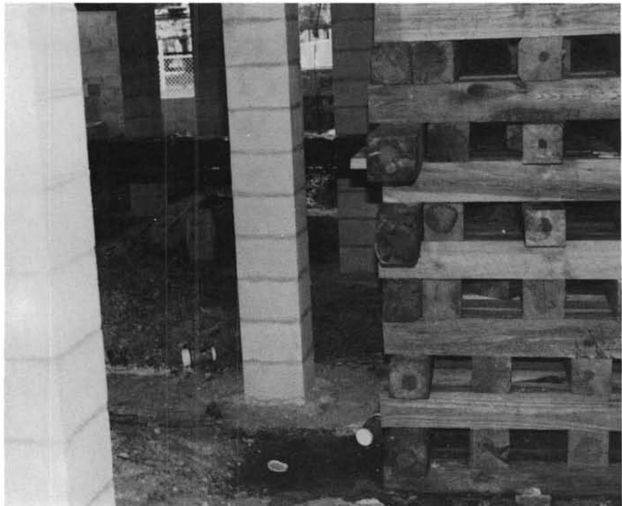
Footings for the piers and perimeter and interior grade beams were poured after the structure was located on the site and raised to the planned elevation.
