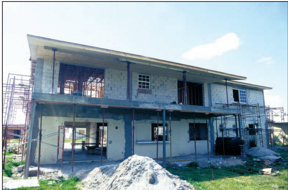
Figure 47 The tiedown columns extend down from the new second-story walls and into the original first-floor walls. The columns tie the first and second stories together and provide a continuous load path that helps the house resist the forces of high winds.
