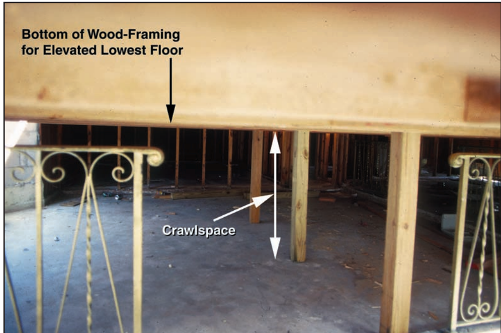
Figure 68 Rather than install a new concrete slab on compacted fill, the owner of this house chose to build a new wood-frame floor above the old concrete slab. This method creates a crawlspace below the new floor.
